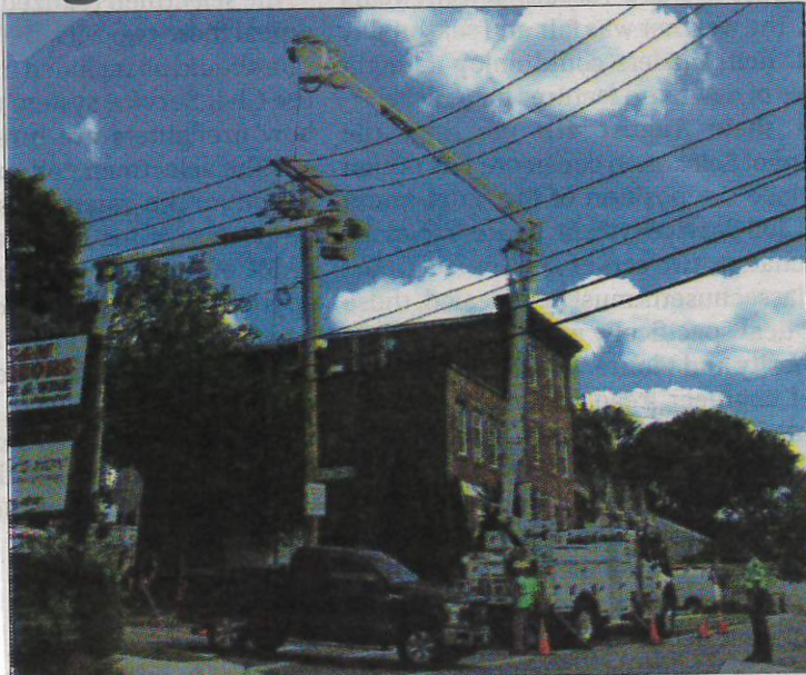
WAKEFIELD MUNICIPAL Gas & Light Department crews worked recently at Water and Preston streets.
